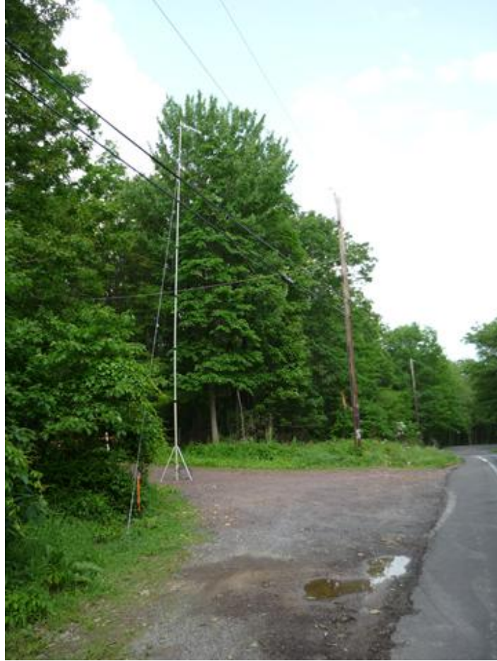
Figure 4: 2011 Weatherly B TLink Antenna Mast
